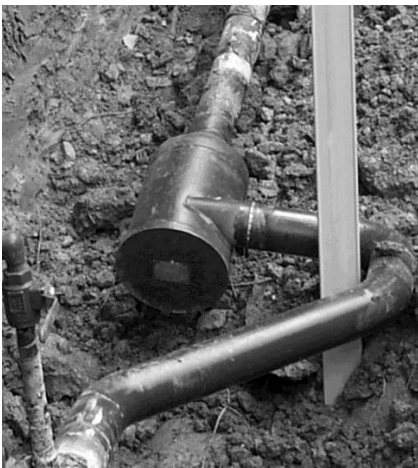
Figure 2: Acceptable install. This is an in-line install with spool in gathering laterals. Note that the inlet is on top.
