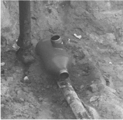
Figure 1: Acceptable install. Installed at a 90-degree angle after a well head (optimal install at the well head).
