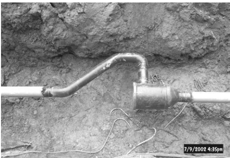
Figure 3: NOT an acceptable install (continued on page 6)
